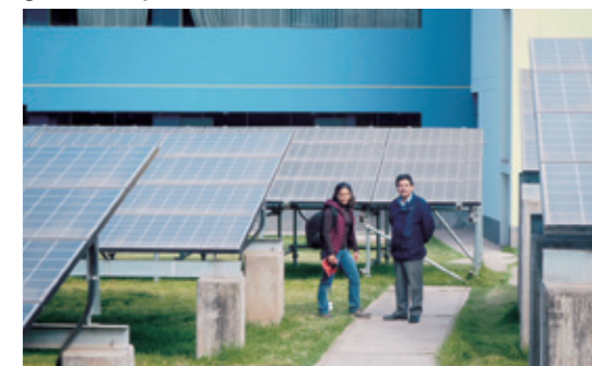
Verification of the usage situation of a solar power generation system (Peru, 2018)
