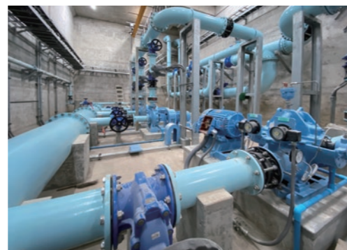
Water piping within the facilities
