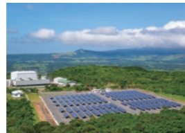
Solar power generation systems
