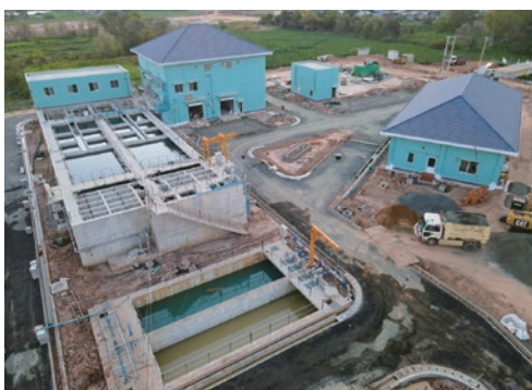
Completed water supply facilities
