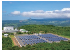
Solar power generation systems
