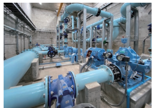
Water piping within the facilities
