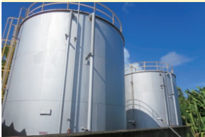
The fuel tank of Tuvalu Electricity Corporation
