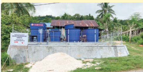
Water purification system installed in a village (Courtesy of Yamaha Motor Co., Ltd.)
