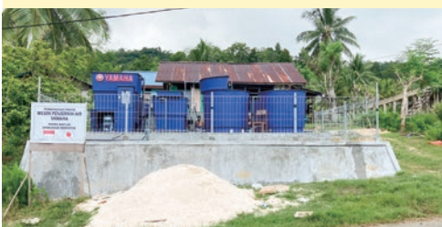
Water purification system installed in a village (Courtesy of Yamaha Motor Co., Ltd.)
