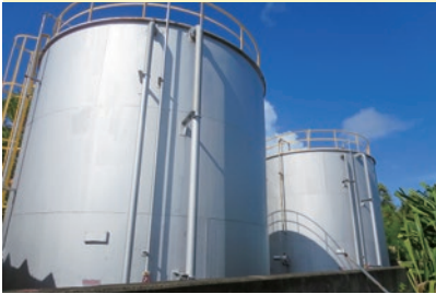
The fuel tank of Tuvalu Electricity Corporation
