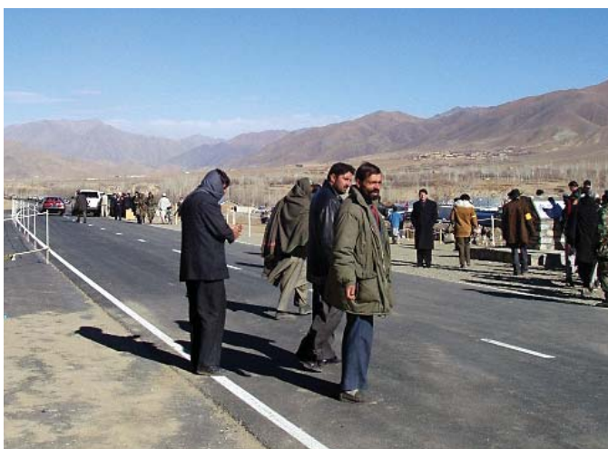
Afghanistan The trunk road from Kandahar toward Kabul built using non-project grant aid
