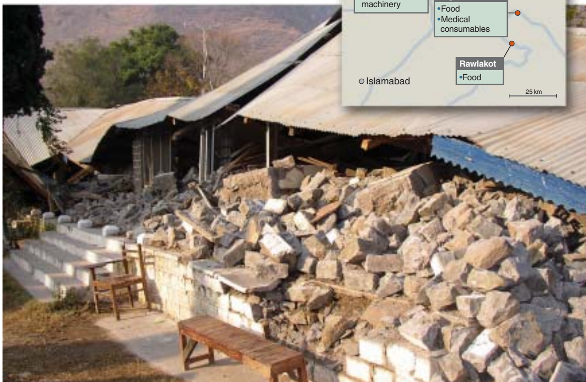
A damaged school, Jhelum Valley
